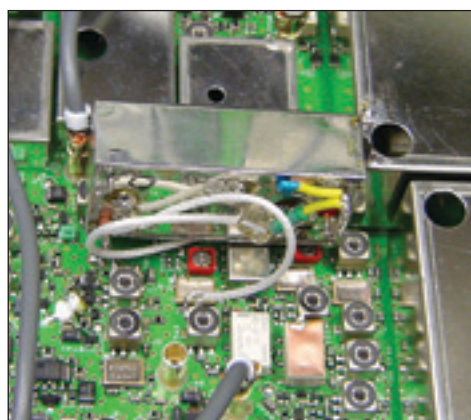
Figure 3 — Initially we installed the filter as shown here. It didn't perform as expected, and we learned that the leads were too long and the capacitor was not needed with our radio.
